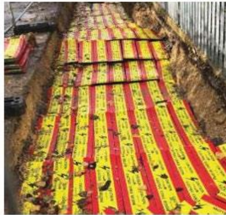
Cable warning tiles
